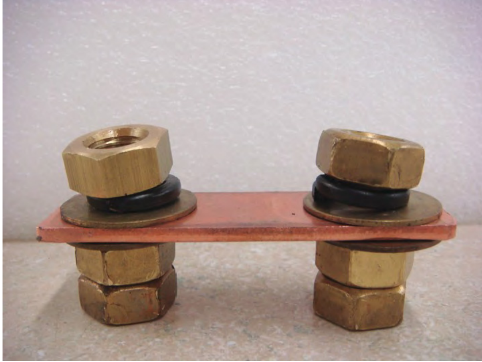
Photo shows extra nuts installed under jumper bar for clearance of power bolt Insulation
